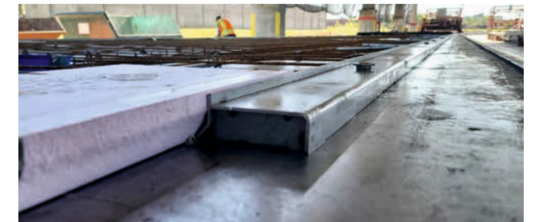
Siderrails for TT slab production are in high demand in the USA
