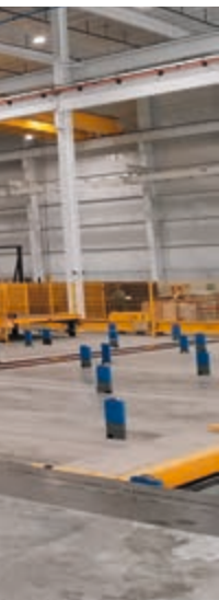
At the tilting station, the finished elements are lifted off and loaded onto transport frames
