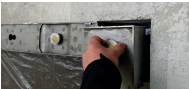
To demould the formwork, only the magnet holder edges are manually lifted out; the side forms are removed by the robot.
