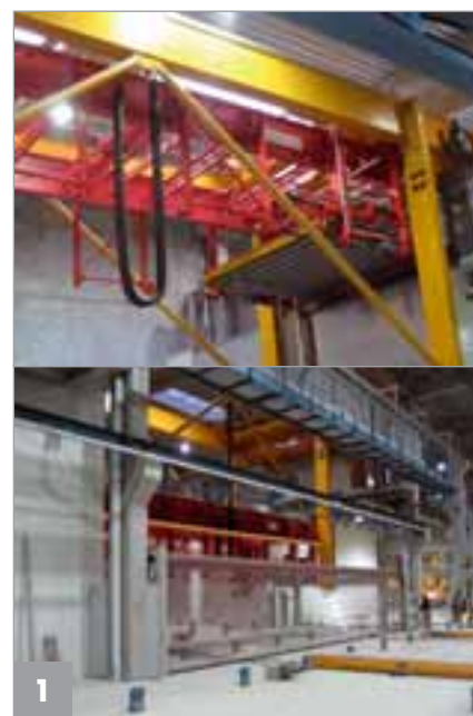
Suspended storage and retrieval system with entrance to hardening chamber
